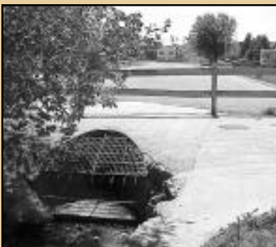
Just add water: Runoff from a summer storm will empty directly from solar-heated roads and rooftops into this cold water feeder stream.
